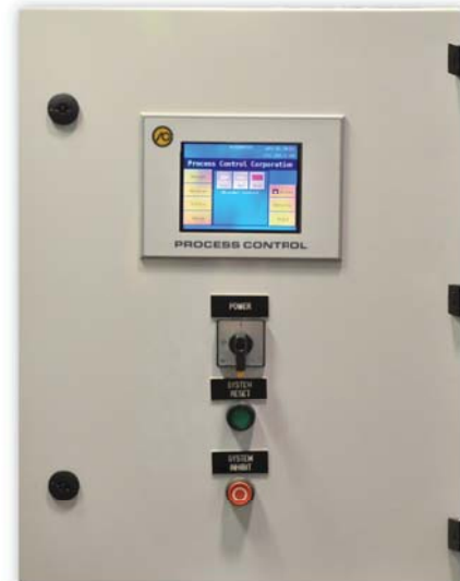
Autobatch Control Panel Upgrade with Color Touch Screen
